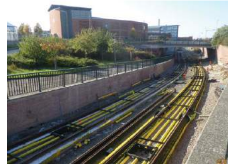
▲ ABOVE: The EMC mitigation system uses feeder cables along the rail, feeding the overhead at each pole.
